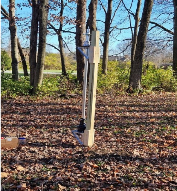
Figure 5 4x4, rotor, and thrust bearing on "tower" portion. Looks crooked but it isn't!
